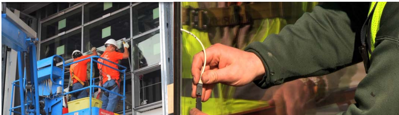
Figure 5: Images of the installation of SageGlass Electrochromic glazing in a curtain wall system. (Left image) Installation of the glass pane. (Right image) Connection between the pigtail and the frame cable.
